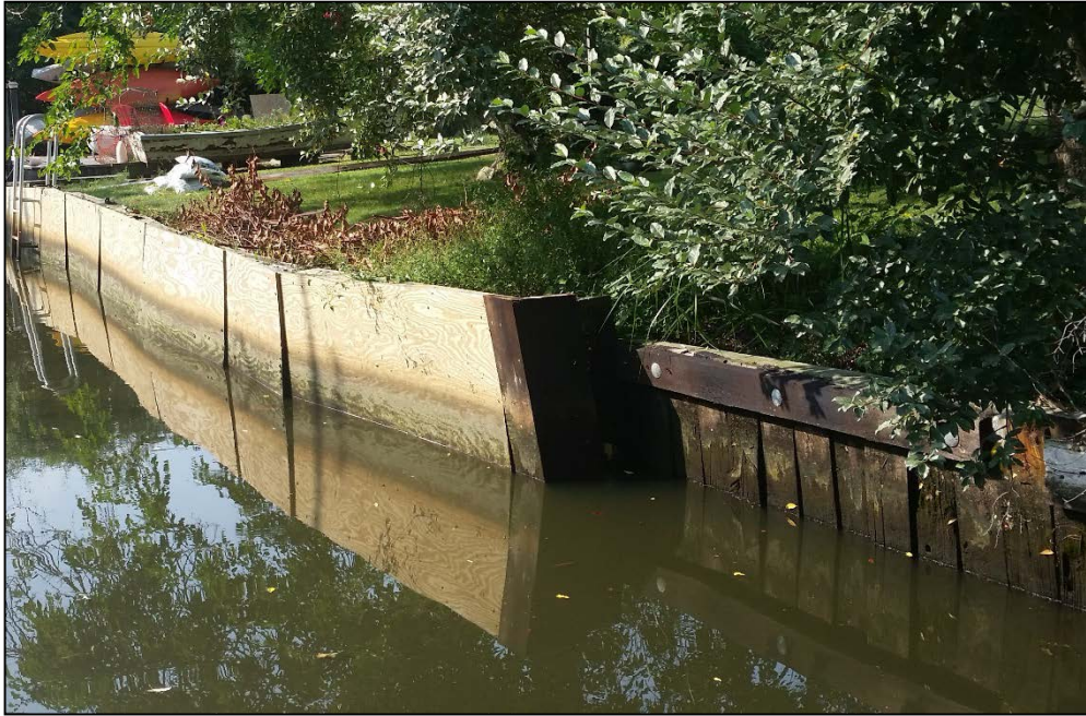
Many bulkheads appear to be vulnerable to failure.
