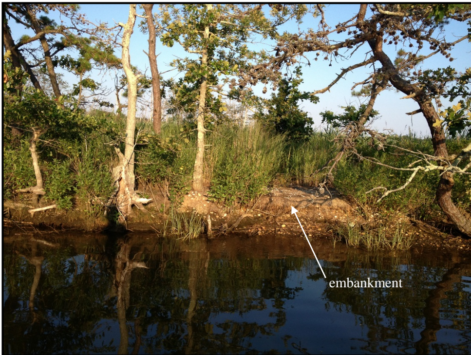
The embankment which separates the canal from the wetland areas is restricted with trees, many of which have exposed roots from erosion.
