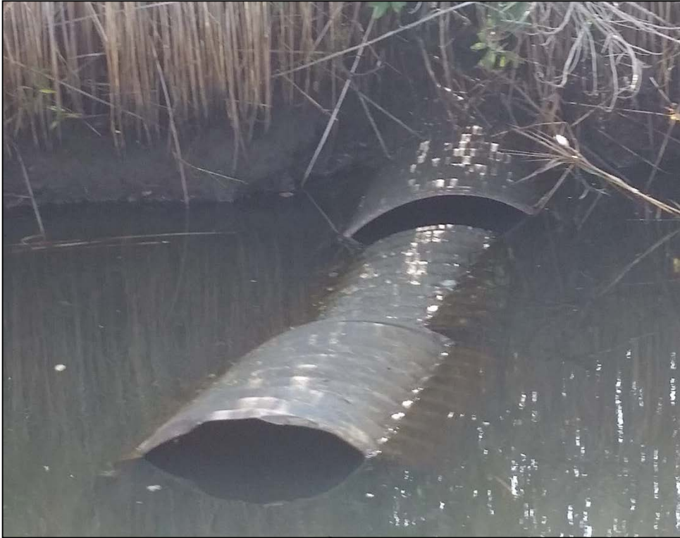
Culverts in poor condition provide little tidal exchange between canal and bermed wetlands.
