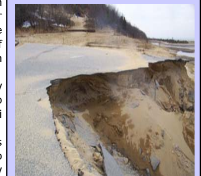
A bluff erosion site in Kings Park, N.Y.
